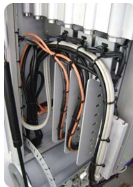
Cable management is integrated for power, networking and KVM.
